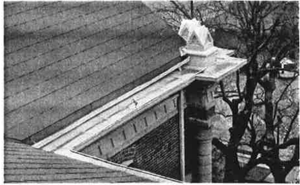
FIGURE III-16. The original gutter was integral to the roof behind a small parapet (the parapet was the same height and profile as the finial base) and drained into internal downspouts in the stair towers. The 1912 gutters are residential style exterior units with an exterior downspout. The dirt on the cornice indicates that it commonly has standing water on it after a rain.
