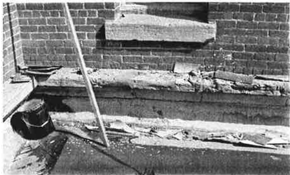
FIGURE III-17. While the annex has red tile roofing on the south and east, the non-visible north and west sides are rolled roofing only. Past repair efforts have left behind a significant amount of debris, most of which can be found blocking the flow of the gutter.
