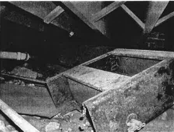
FIGURE III-12. The crawlspace is a jumbled array of active and abandoned utility equipment, original construction debris, and everyday trash. The 2x14 joists and cross bracing appear to be in good shape.
