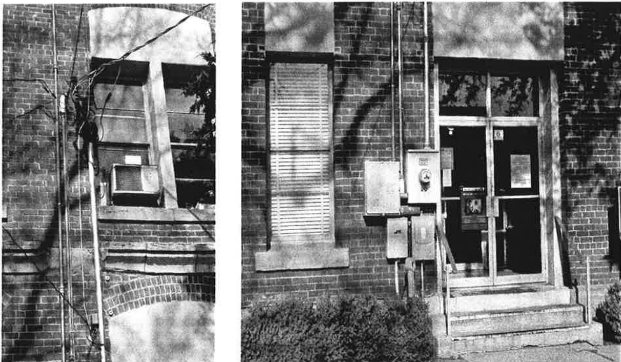
FIGURE III-38. As part of installing the weatherhead, a portion of the stone belt course was removed (left). The resultant installation has an extremely negative impact on the visual aesthetic of the east facade of the courthouse, as visitors are forced to enter the building in close proximity to the equipment (right).
