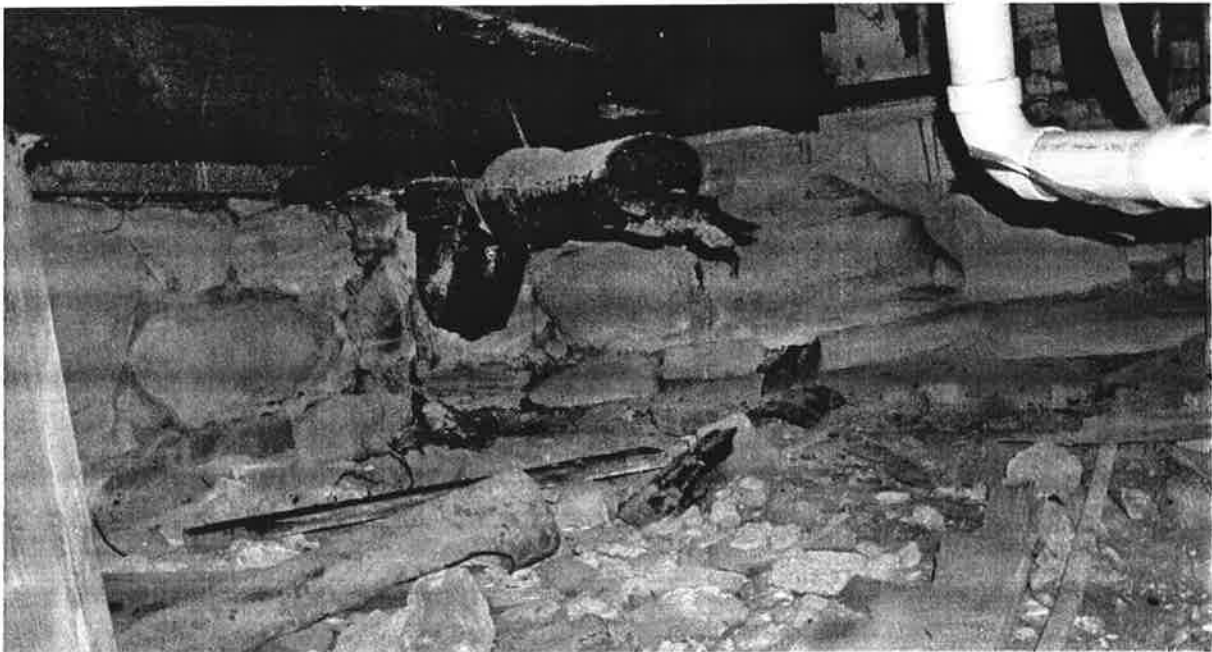
FIGURE III-6. The foundation sandstone is in relatively good condition. However, evidence of rising damp can be seen in the form of efflorescence on the mortar and in the piles of fine dust (degraded mortar) at the base of the foundation walls. Loss of mortar integrity is a serious problem affecting the future stability of the building.
