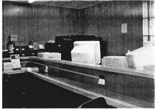
FIGURE III-11. The image above illustrates the typical office condition. Wood paneling covers the walls from the base to the acoustic tile ceiling. A non-original counter can be seen in the foreground.
