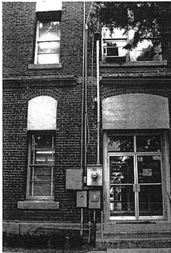
A myriad of detrimental changes exist on the building exterior, including aluminum doors and windows that do not fit original openings, surface mounted conduits, and damaging alterations to the masonry. (Photo from THC files)
