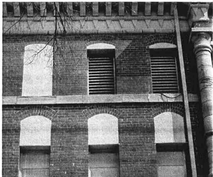
FIGURE III-25. This image shows all of the various window treatments currently existing. Most third floor windows are fully blocked. Only a very few have been converted to louvers. The remainder of the windows have been only partially blocked. The blockage corresponds to the location of the ceiling inside the building. Also, by filling the arch, the replacement windows could be cheaper, standard units.
